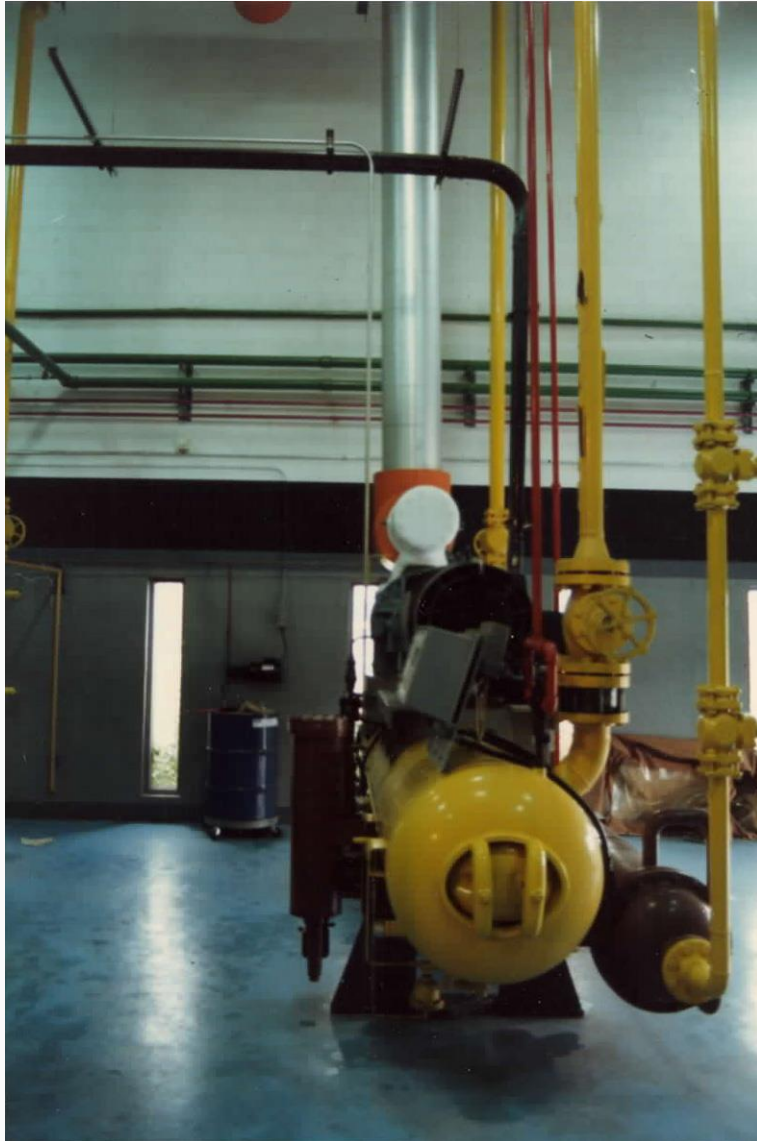
First Thermosyphon Oil Cooling System Installed -- Attalla, AL
