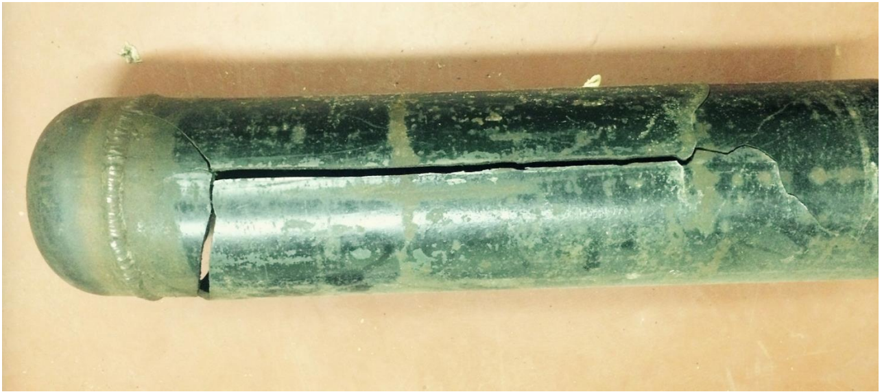
Broken pipe due to critical sonic flow, caused by a CK-2 that failed open.
