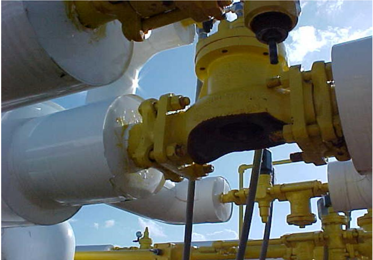
CK-2 valve that failed open, causing a liquid cannonball.
