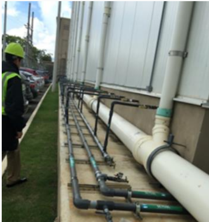
Glycol Underfloor Heating System
