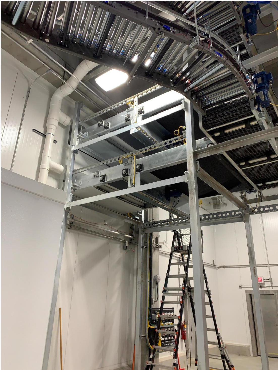
Example of a good location for a desiccant unit -- spiral freezer outfeed.
